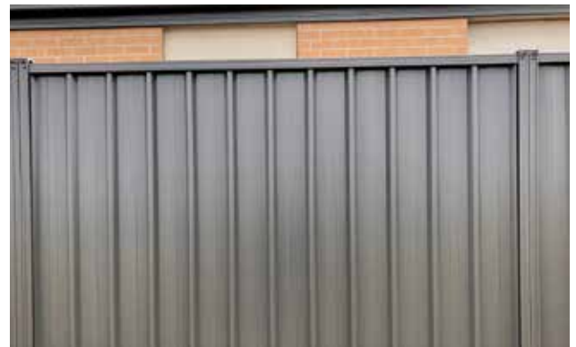
PHOTO 2 Internal boundary fencing : pre-painted steel in Woodland Grey colour
